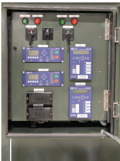
First Door Open Revealing Door Mounted Equipment Used For Normal Operation
